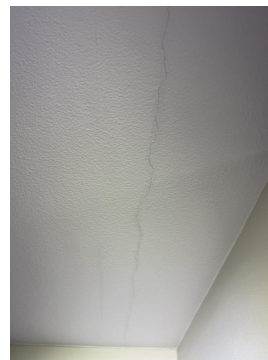
Riss i betong himling/etasjeskille.
