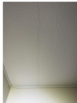
Riss i betong himling/etasjeskille.
