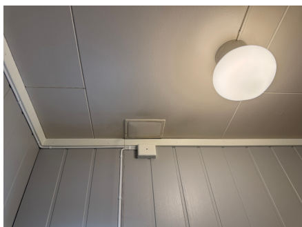
Ventil montert i himling
