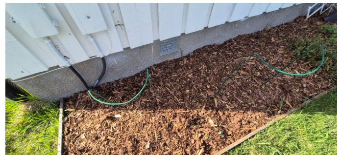
Mur under peisestue
